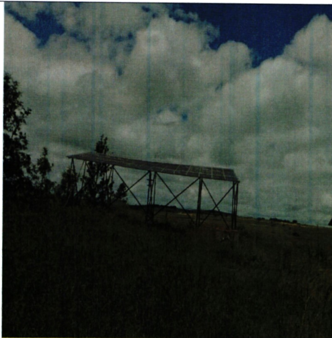
Solar Power water pumping system in Narok
