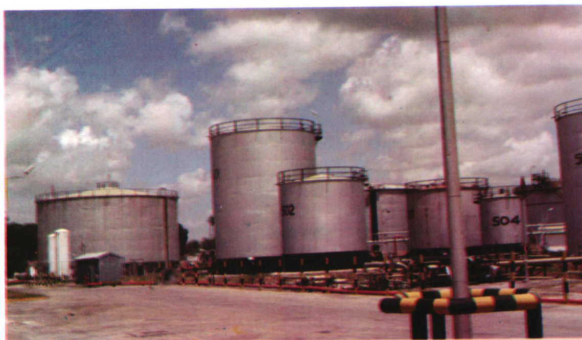
Part of the Kenya Petroleum Refineries complex at Changamwe, Mombasa.
