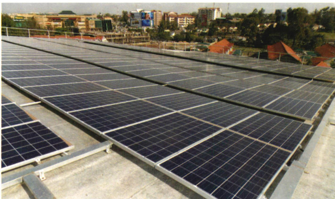
Solar photovoltaic panels at a university in Nairobi.
