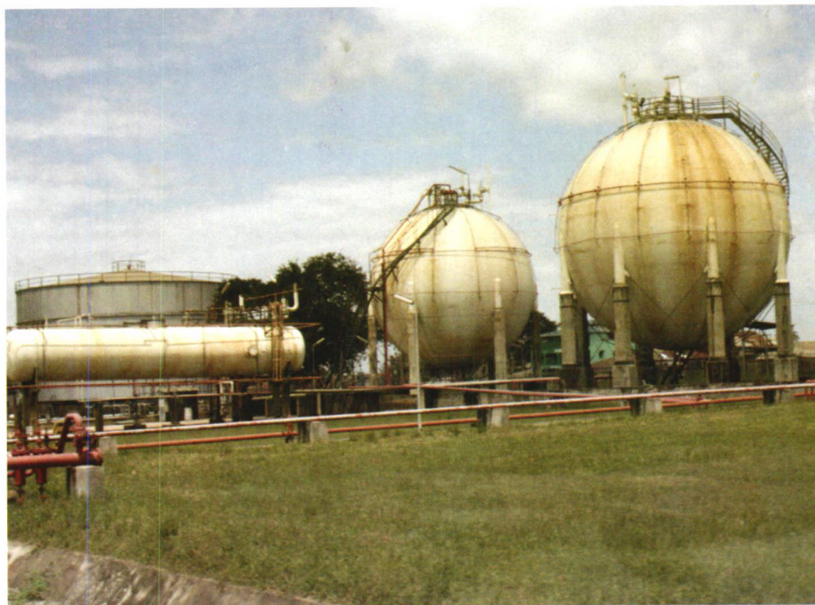
Petroleum processing and storage facilities at the Changamwe Oil Refinery, Mombasa
