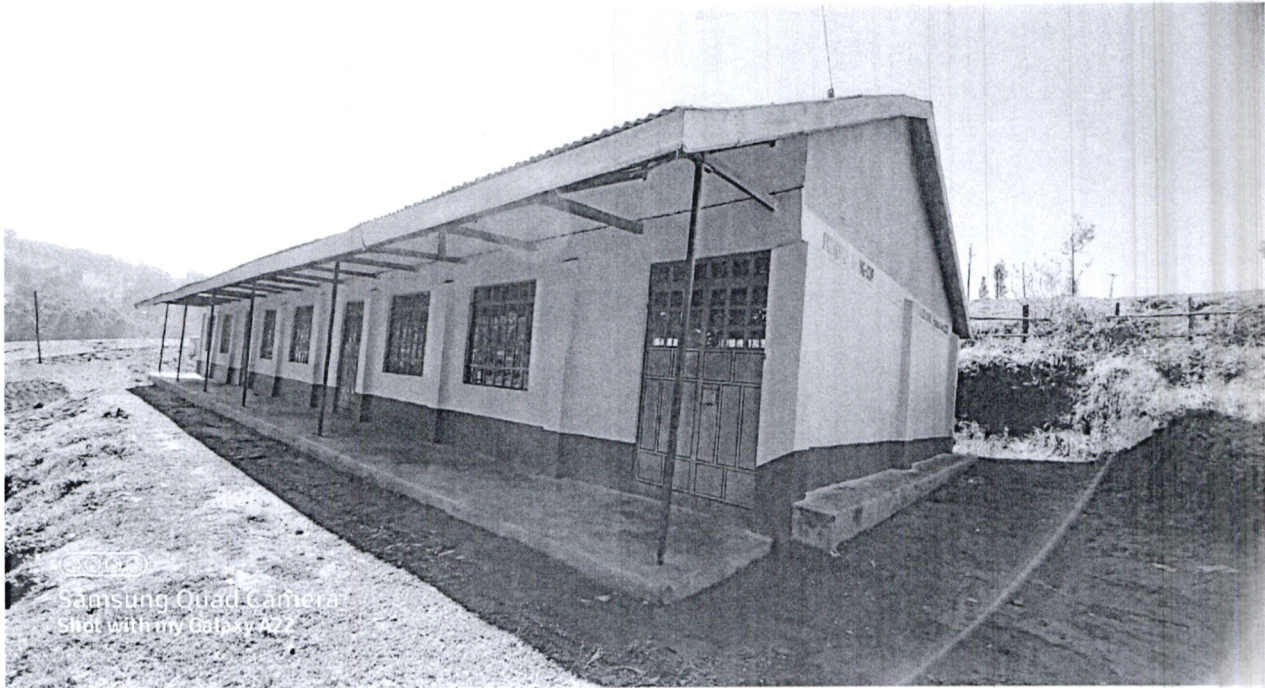
Construction of three class rooms at Masige Primary school at a cost of Kshs 2,700,000.
