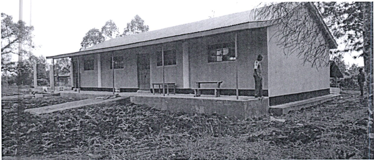
Construction of two class rooms at Saiga Ngiya Primary school at a cost of Kshs 2,000,000.
