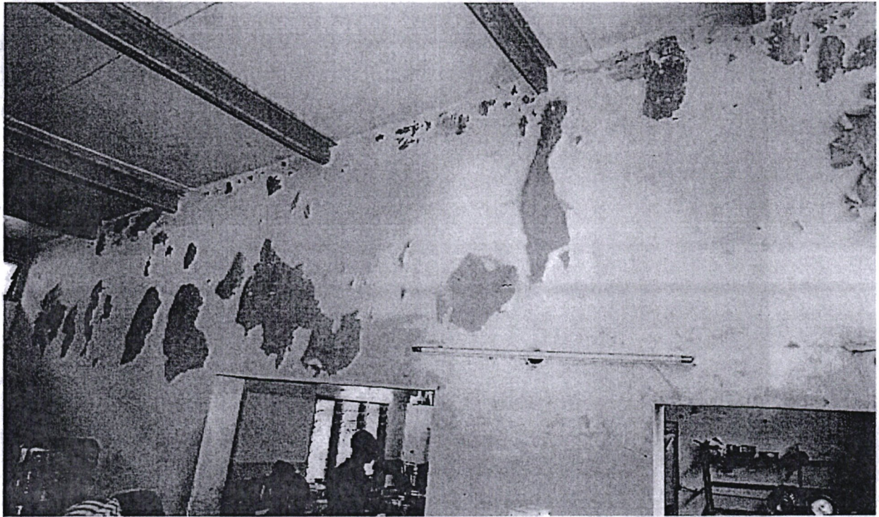
Picture 4: The Committee observed widespread infrastructural deterioration with worn-out floors, walls and peeling paints witnessed in majority of the hospital wards visited.
