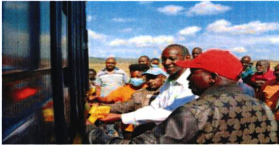
Prof. Ikua cuts tape to officially signify the commencement of mini-grid installation. He is flanked by Chief Kipees to his left, Mr. Cherbogei and REREC’s Purity Kimotho to his right.
