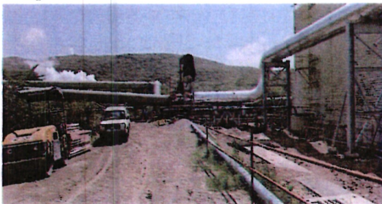
Steam pipes at 83MW Olkaria I Unit 6
