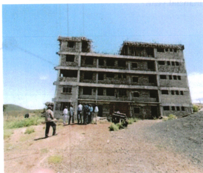
Ongoing Construction of Marsabit High Court from the side and some materials on site
