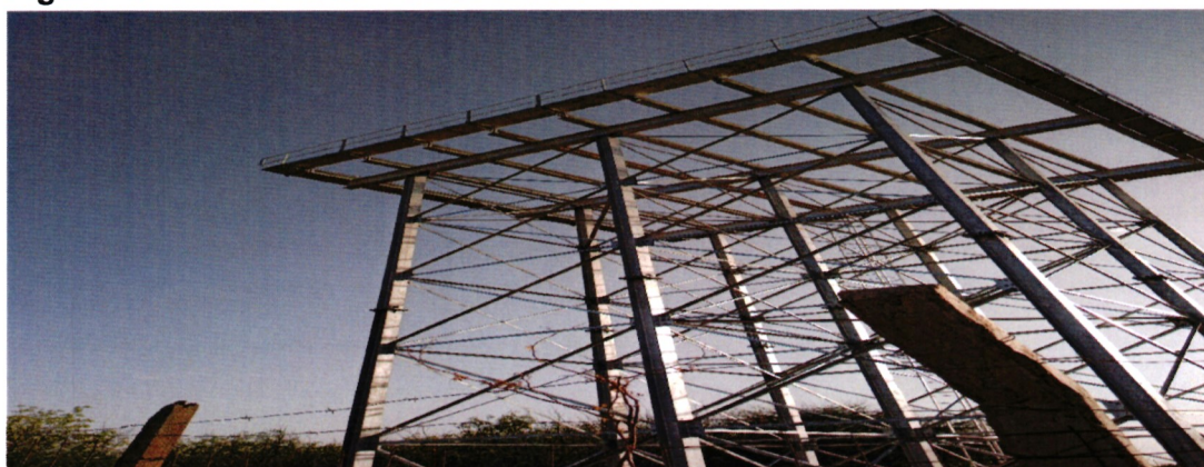
Figure 4: The 15 Meter Tower Where a 300m 3 Steel Tank Was to be Placed
