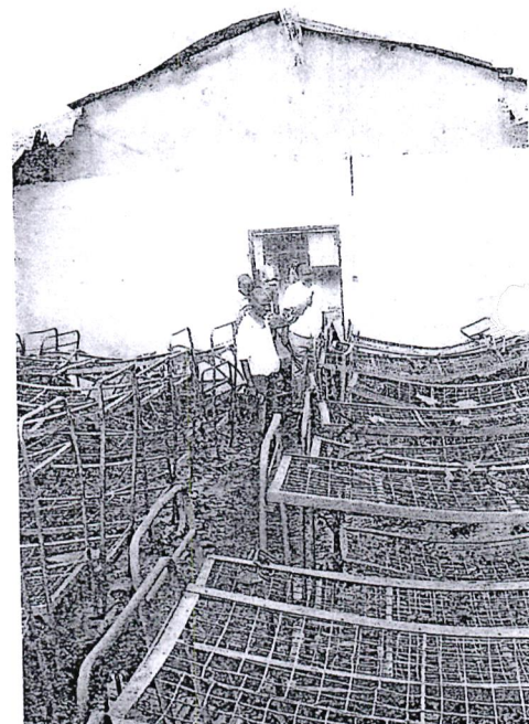
File. This is what was left of a dormitory in Njoro Girls' High School after a fire incident on Saturday. The cause of the fire was by yesterday yet to be established. [Kennedy Gachui, Standard]
