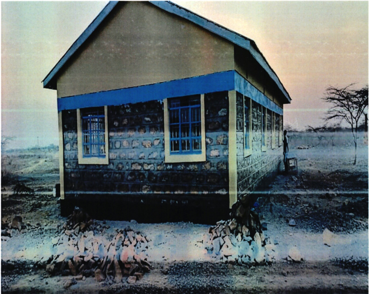
PROJECT: CONSTRUCTION TO COMPLETION OF FOUR ROOMED OFFICE AT KAIKOR ASSISTANT COUNTY COMMISSIONER'S OFFICE, FINANCIAL YEAR 2022/2023
