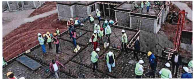
His Excellency The President interacting with the construction workers during one of the site visits.
