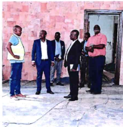
NHC management led by Managing Director/ CEO Qs. David Mathu and General Manager- Construction & Project Management Eng. Thomas Ofwa inspecting the renovation work at the Deputy Chief Justice office.
