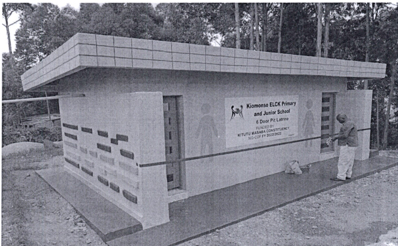
2. Kiomonso Primary School- Construction of 6 door modern toilet at a cost of Kshs. 1,100,000 million
