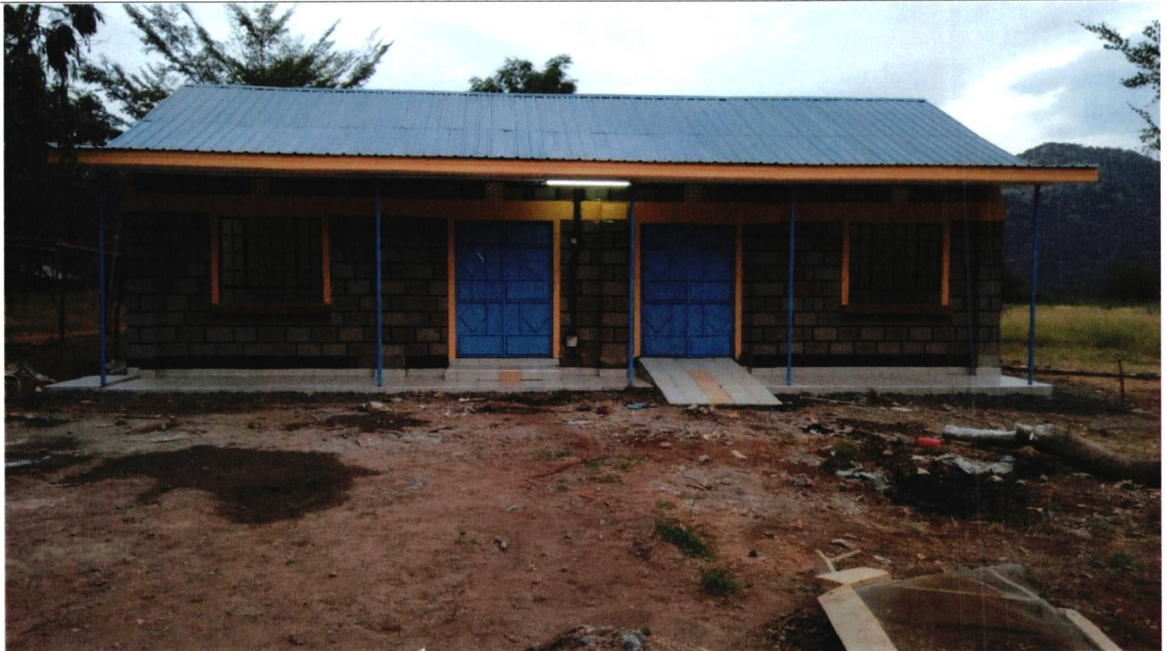
Figure 2: New Administration Block constructed by KMFRI for Mutonga Primary School in 2019/2020 FY
