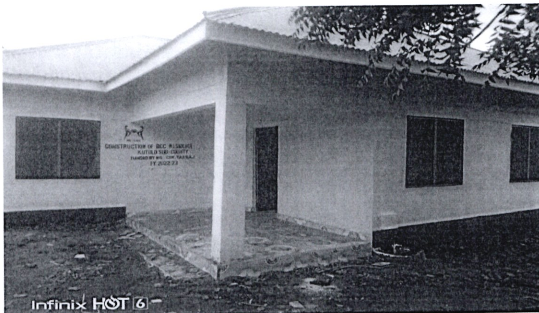
Construction of Kutulo Deputy Sub-county commissioner's residential quarter comprising of 2 bedroom, sitting room, kitchen, bathroom and store.
