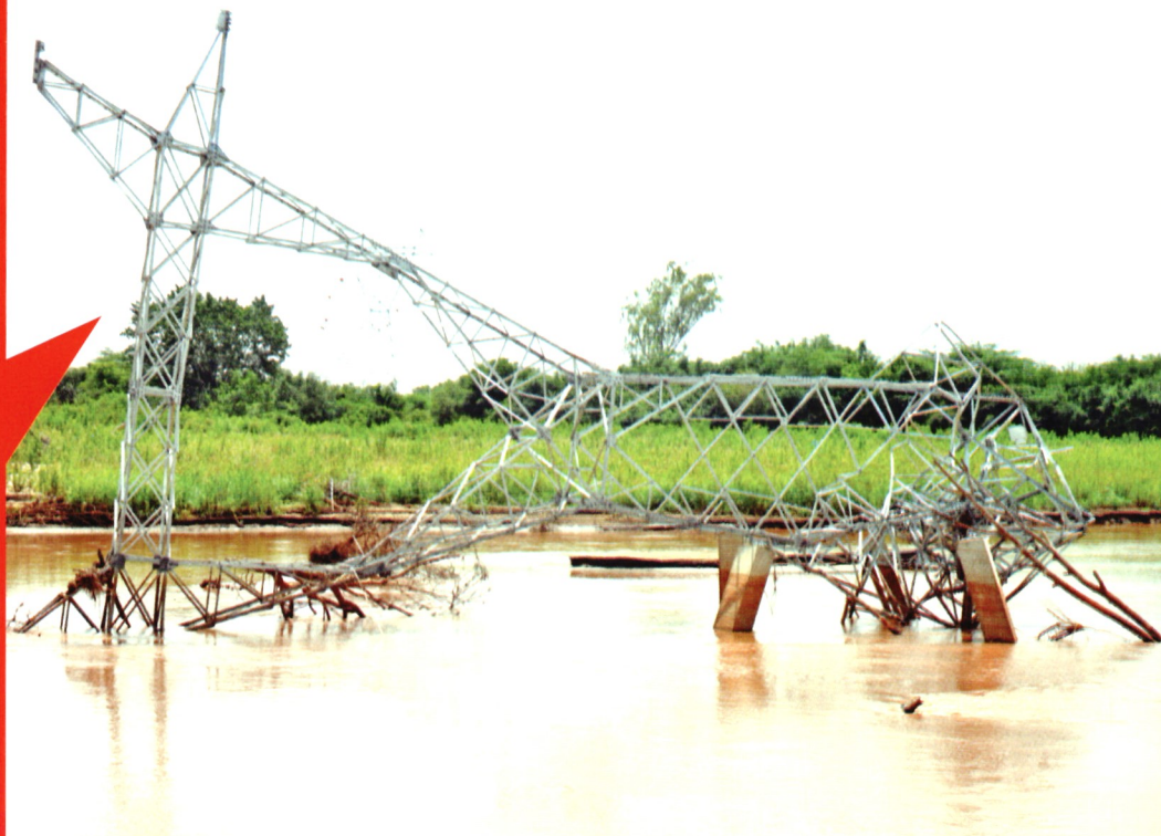
River Sabaki floods collapse tower along the Rabai-Malindi-Garsen-Lamu Line
