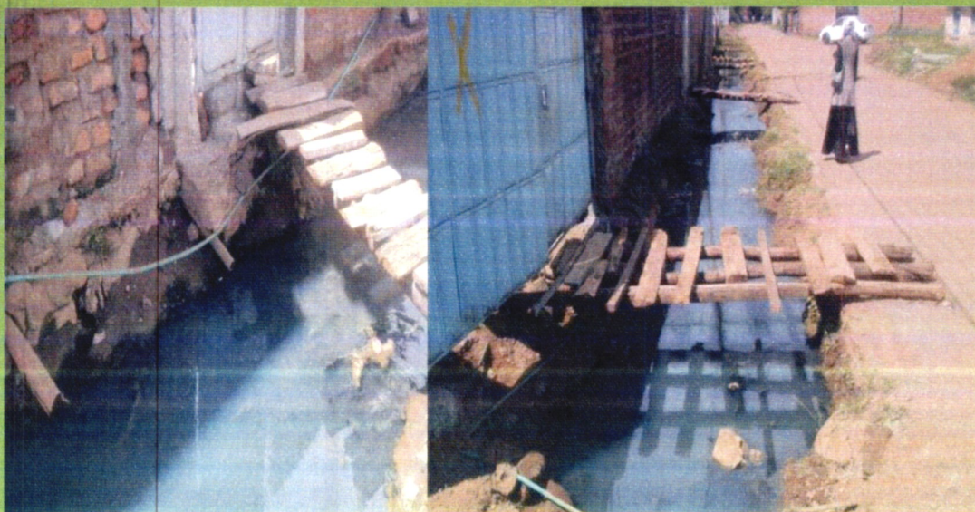
Notice the discharge of raw sewage from the residential units forming a stream of sewage in storm drains hence posing a serious health hazard to residents of Lower Migosi and the neighbouring estates.
