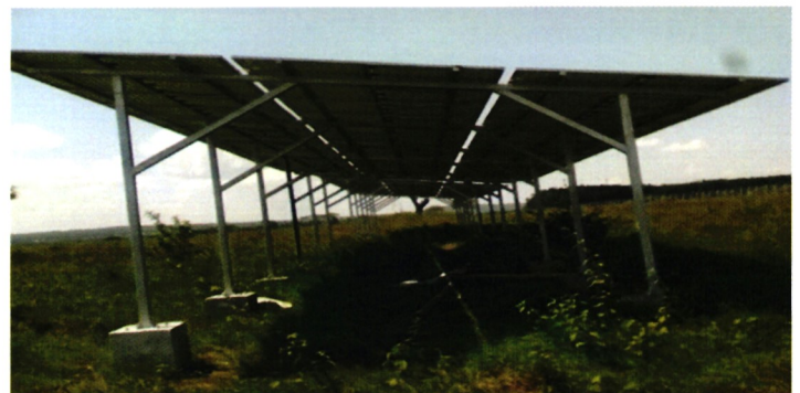
Solar panel array in Alupe
