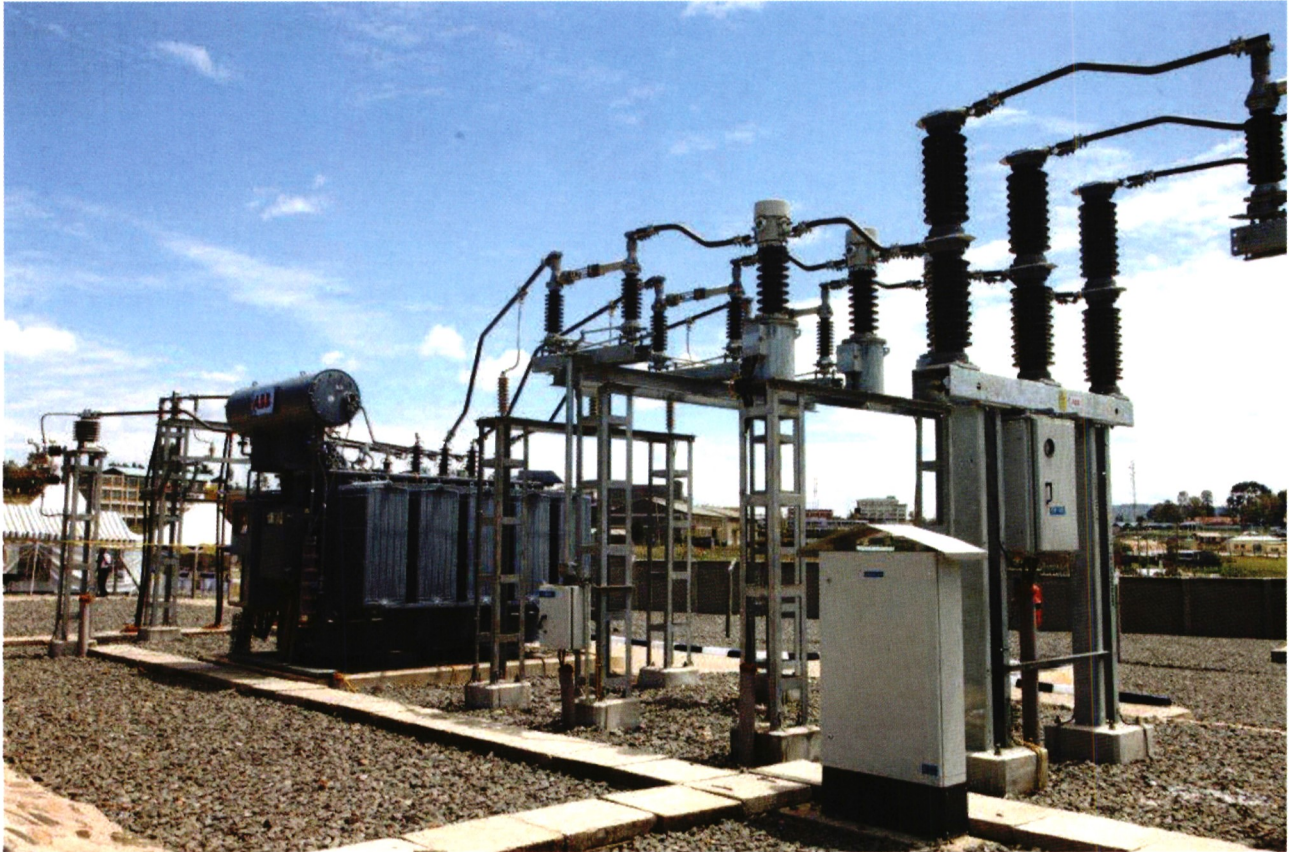
Bomet Substation during its commissioning.
