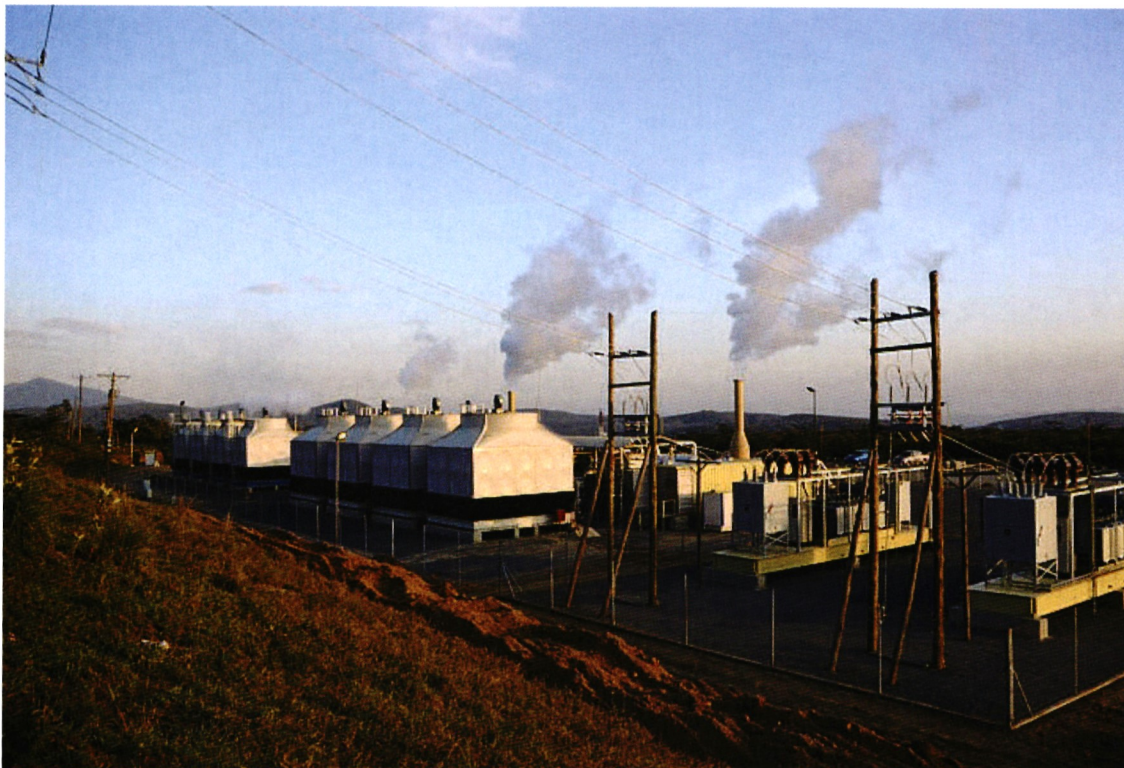
70MW Geothermal wellhead Project
