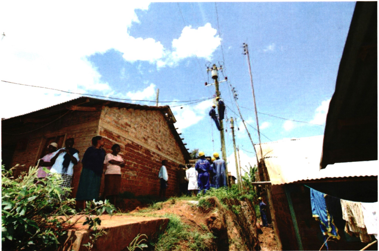
Kenya Power technicians prepare to install electricity to a house in Majimbo, an informal settlement in Embu County in April 2013.
