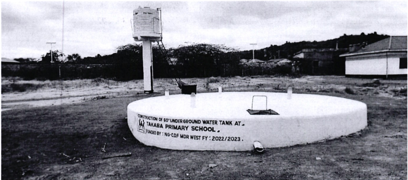
Construction of underground water tank at Takaba Primary and Junior School. This provides much need water storage and improves access to clean water
