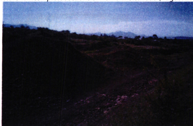
Picture 1: Incomplete sections of Homa-Mbita road (August 2014)
