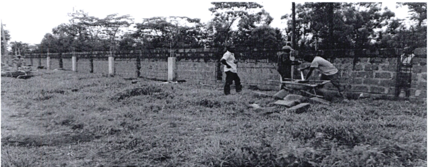
Figure 8: Construction of the College Perimeter wall to enhance security and safety of its property at Ksh 250M.
