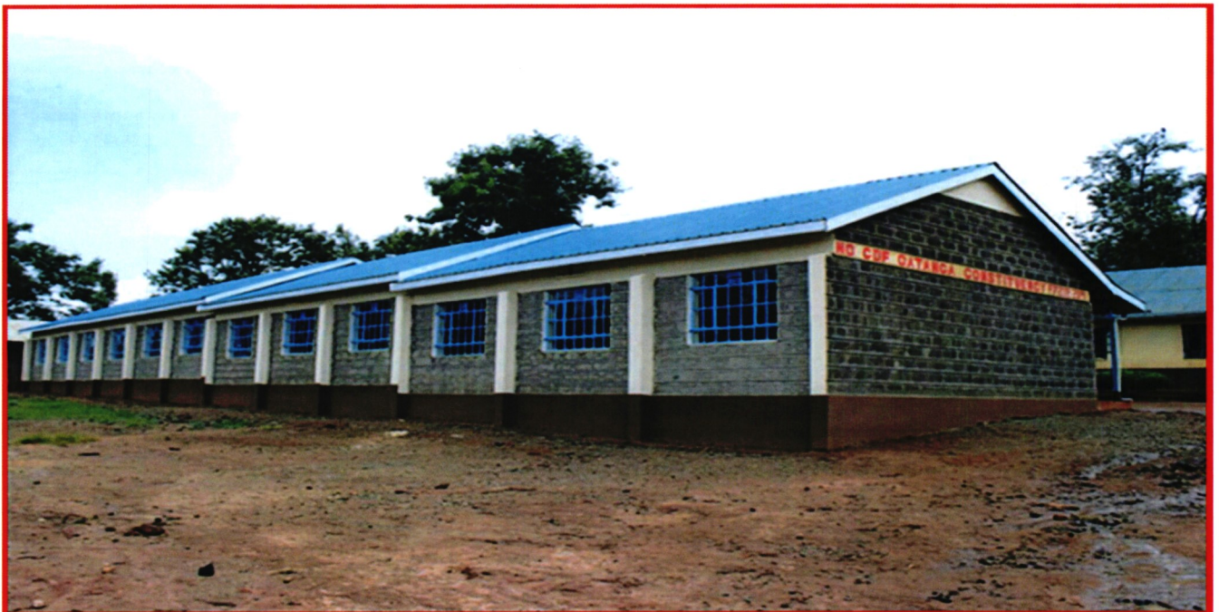
Construction of four Standard Classroom at Ngatho Primary School (The project expected to provide a 160 pupil learning space each year and 120 pupils learning space where COVID-19 is concern)
