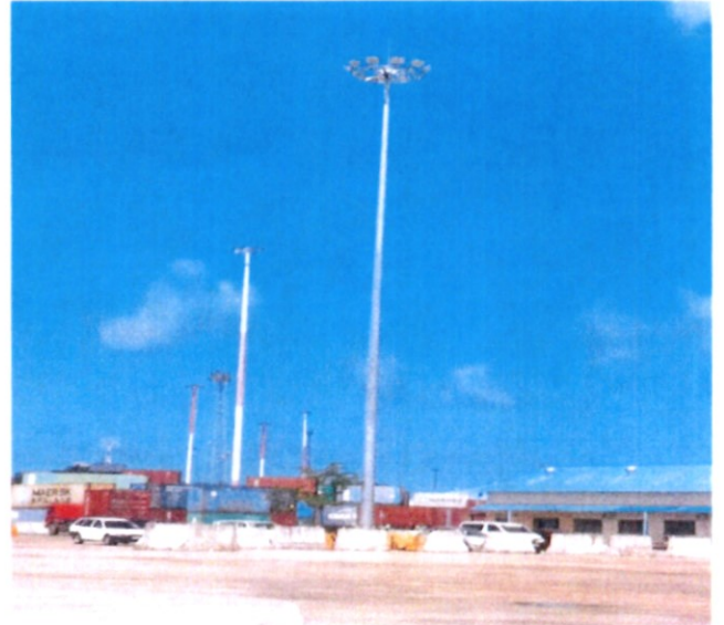
LED YARD LIGHTING
