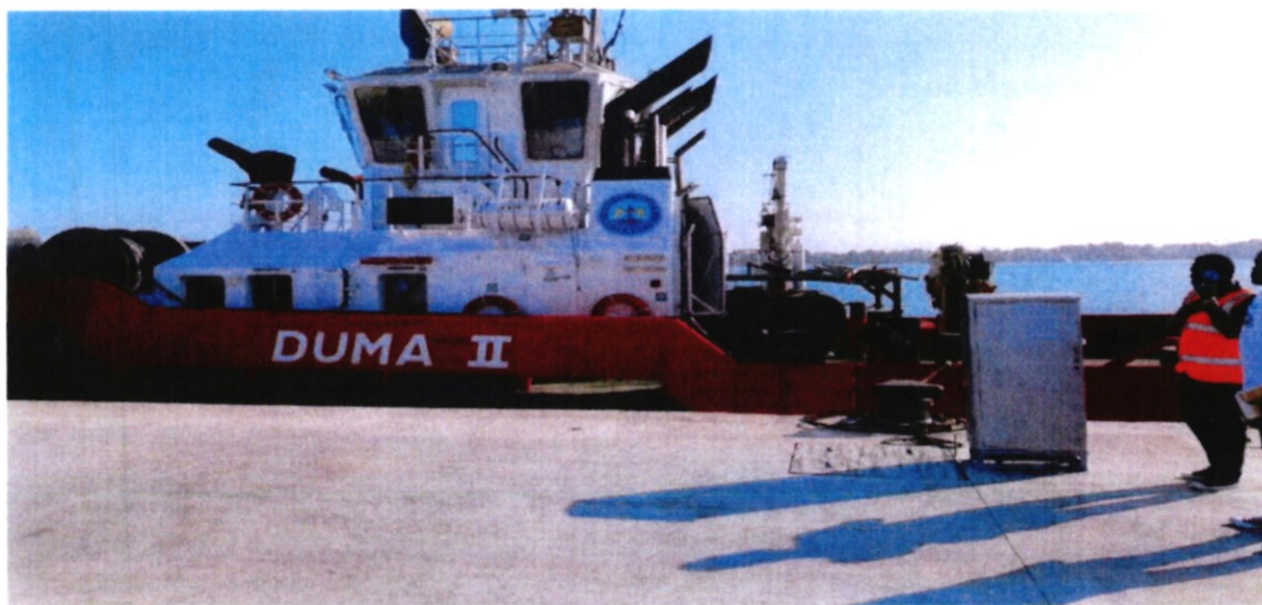
Tugboat jetty at dock yard fitted with shore power boxes
