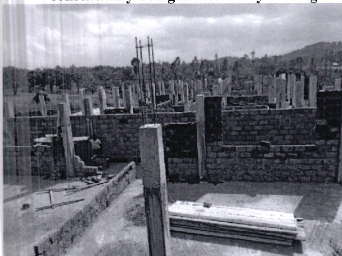
Construction of proposed Uriri Technical and Vocational college in Uriri constituency, being mentored by Mawego TTI on behalf of Ministry of Education
