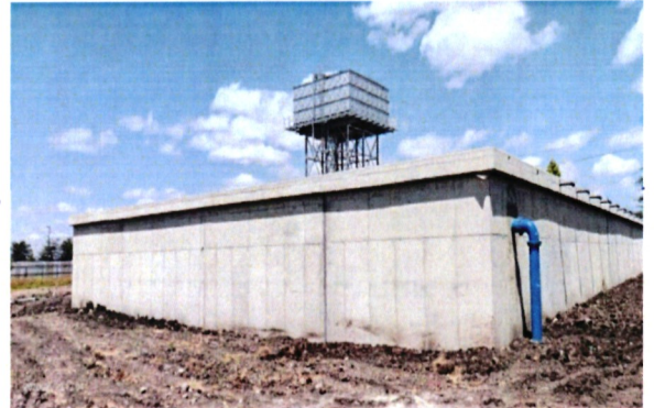
Mavoko Drinking Water Project- Syokimau_4000m3 Reservoir
