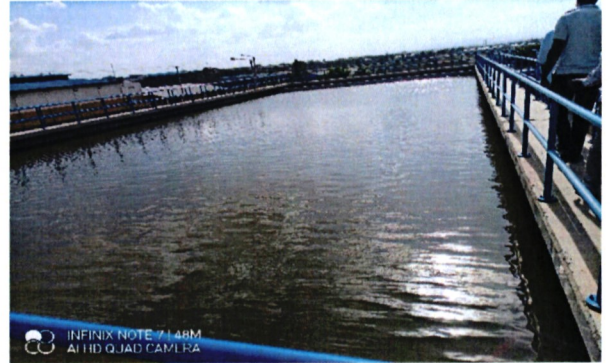
Mavoko Drinking Water Project Water Treatment Plant- Pre-settlement Tank
