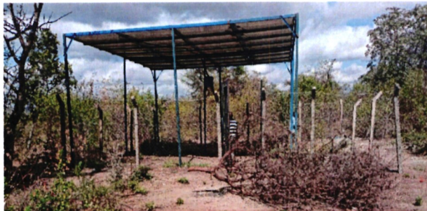
Borehole equipping using solar technology to cut on electricity cost
