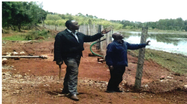
Overview of the Sama Mariki project showing the reservoir, fence and irrigation pipeline
