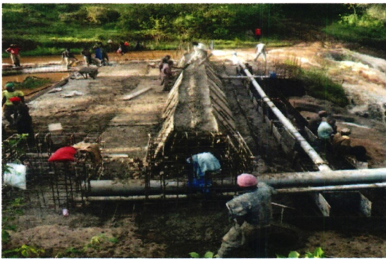
Gaitega Gatari Small Holder project water intake structure and pipeline installation works
