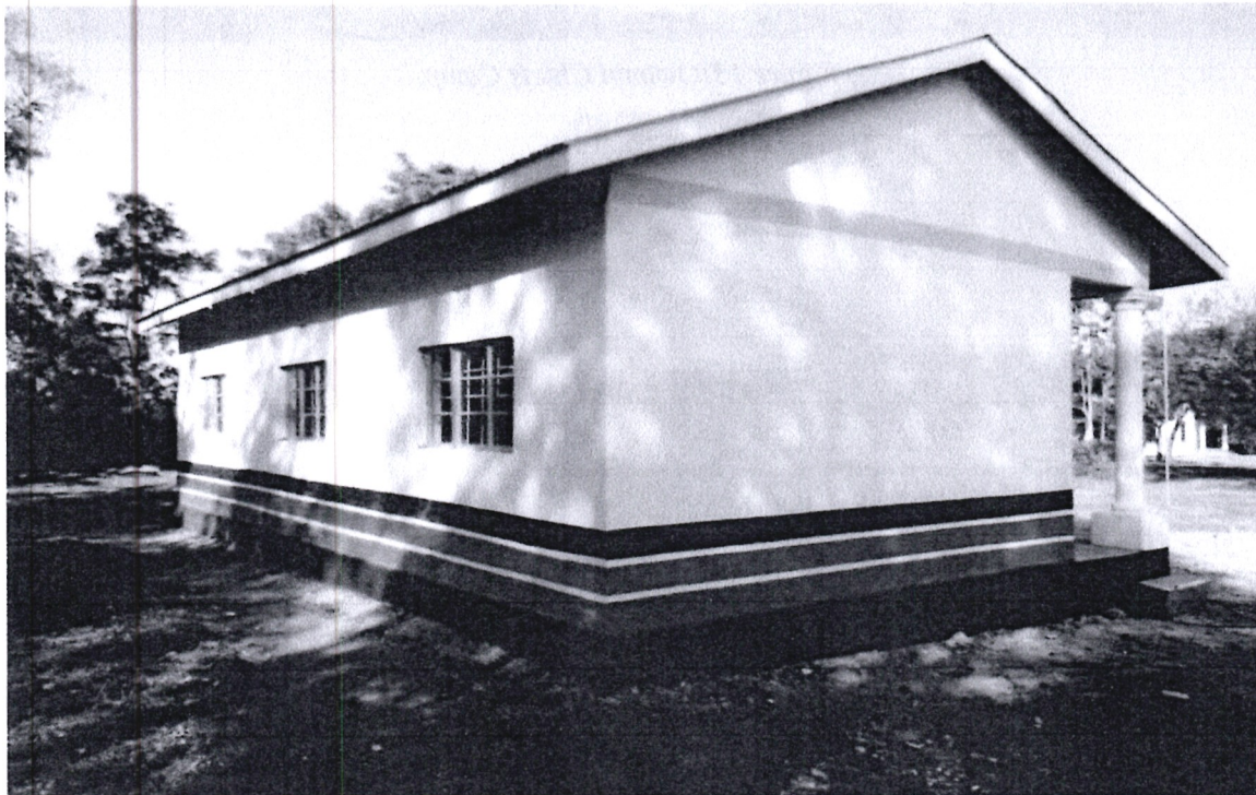
Figure 12: Renovation of 3 roomed chief's office to completion: Replacement of old roof, repair of wall, windows and doors.
