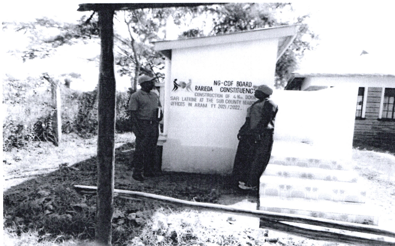
Figure 4: Construction of a 4Number Door Pit Latrine at the Sub County Offices in Aram.
