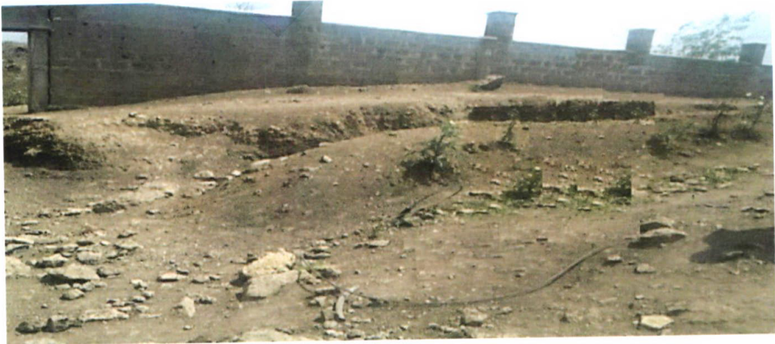
Picture 1: Athi River -Namanga damaged NOFBI phase I section that was not commissioned Source: OAG
