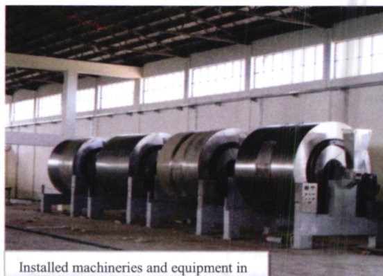
Installed machineries and equipment in ENSDA's leather factory
