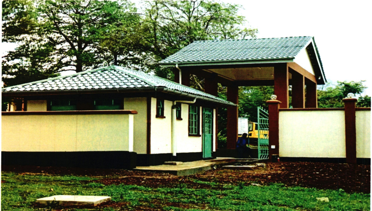
Figure 5: The College main gate under construction at Ksh 5.5M . The new College main gate will enhance the image of the College and improve on safety.
