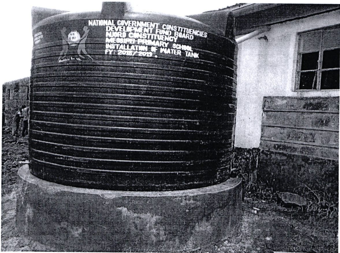
FIG 1.1: INSTALLATION OF WATER TANK FOR WATER HARVESTING AND FOR WATERING TREE SEEDLINGS
