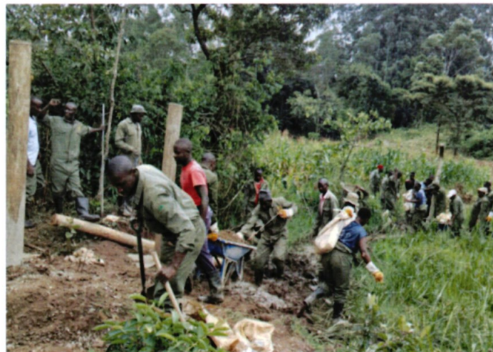
Fencing works ongoing at Shikhusa section, Kakamega Forest. Community members were engaged for the work.
