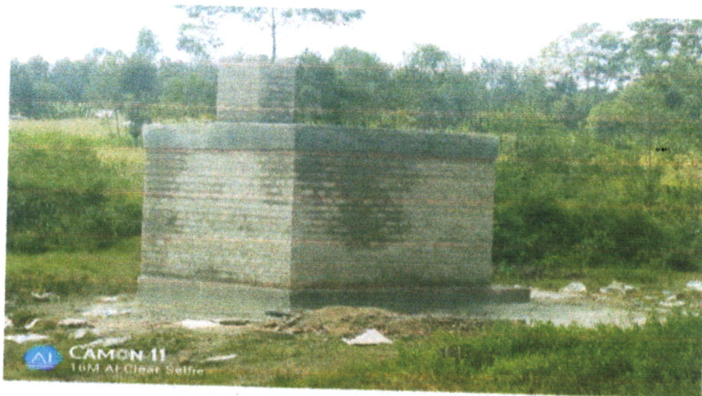
The incinerator/ Burning chamber.
