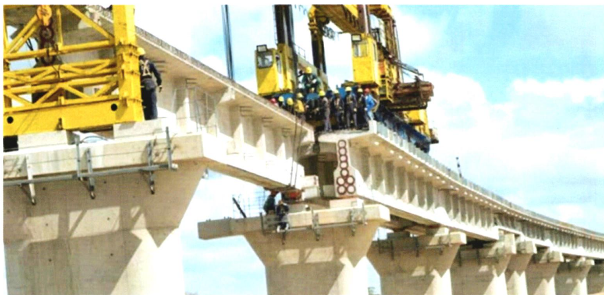
On going construction of the Mombasa-Nairobi railway overpass at Taru – (Mombasa-Nairobi standard gauge railway (SGR) is over 75 per cent complete, with the project expected to be done by December)
