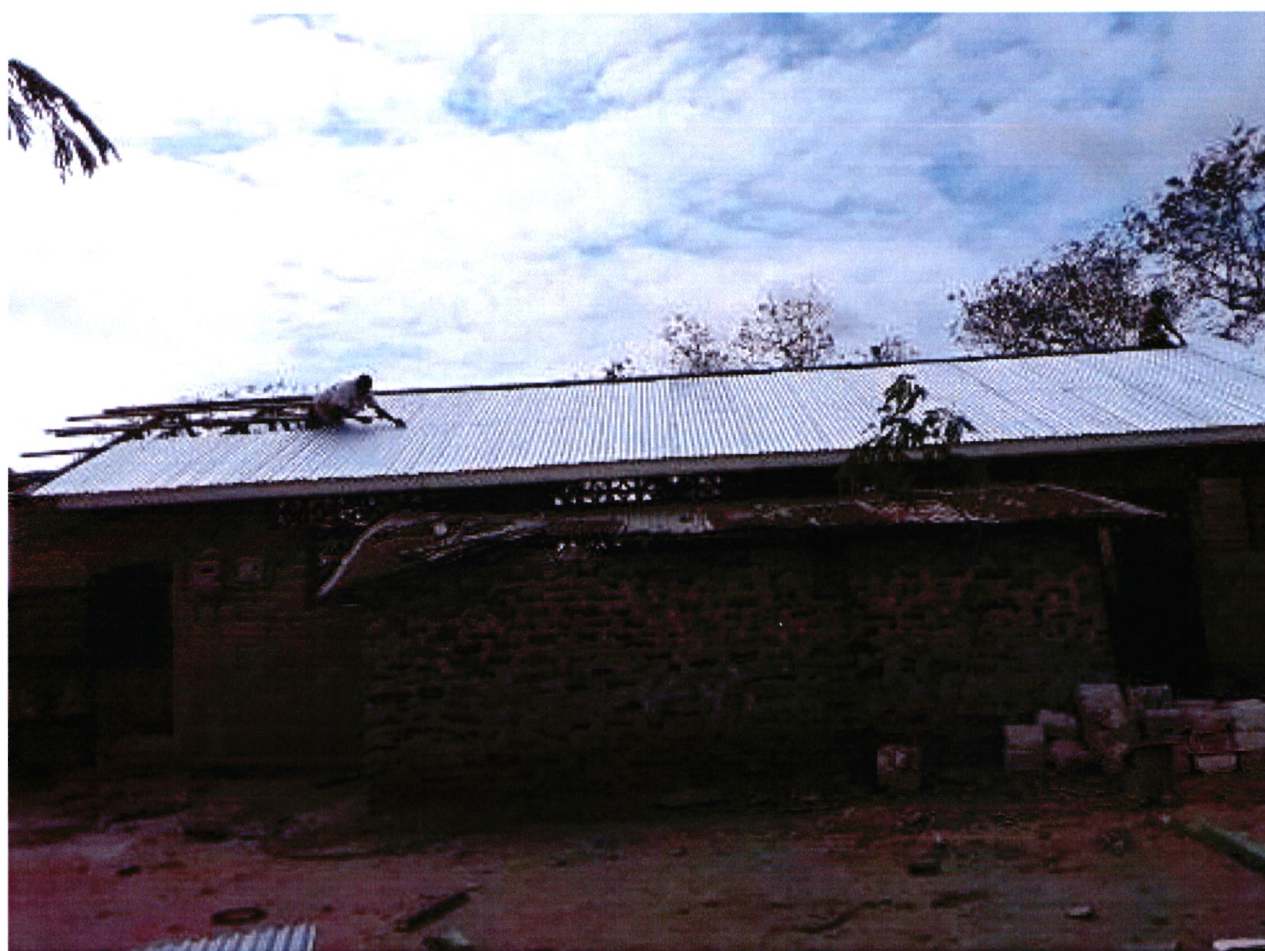
Top: Reconstruction of one of the destroyed roofs at Mtaa Primary School Above: completed roof
