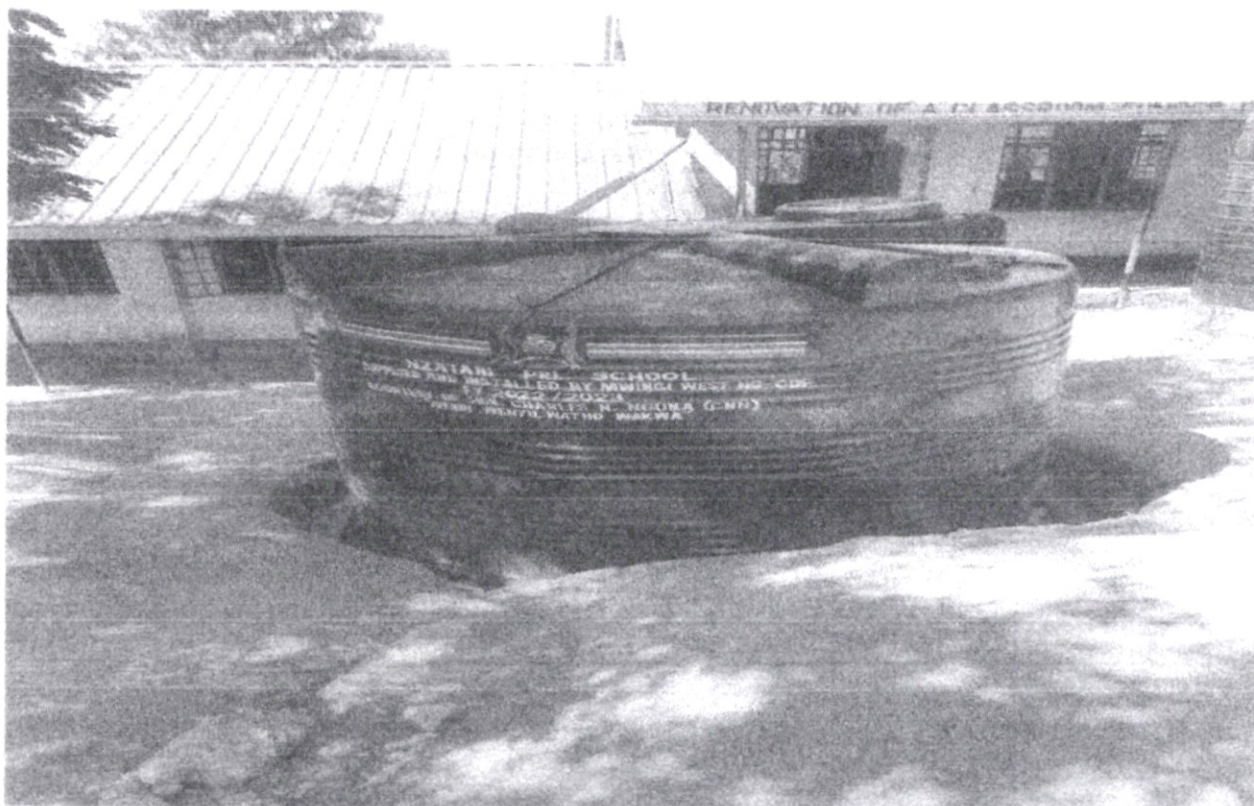
FIG 1.2: Installation of 10,000lt plastic water tank to harvest rain water in Nzatani primary school FY 2022/20223 to boost water storage.
