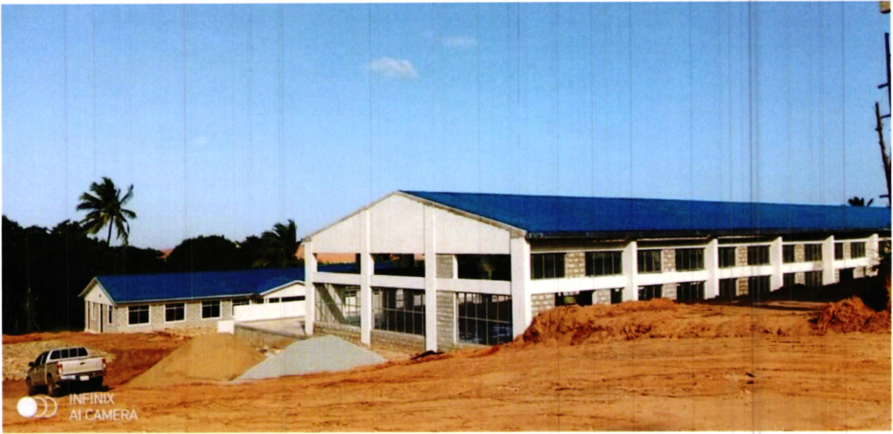
Shimba hills fruit processing plant
