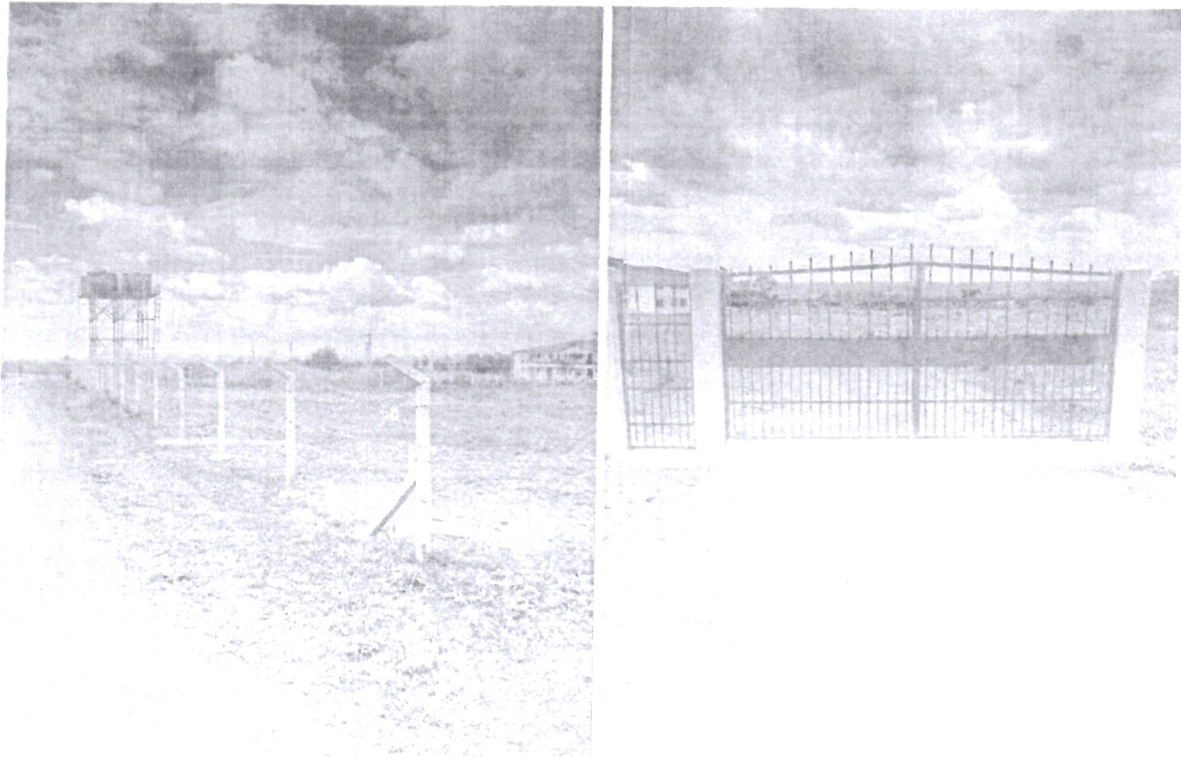
Fig 3: Shows a newly constructed fence, borehole and construction of pipeline and two elevated tanks with a capacity of 10,000 litres at Dr. Daniel Wako Technical Training Institute financial year 2019 – 2020 Matayos Constituency for enhancing learning environment.
