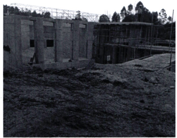
Intake main gate
