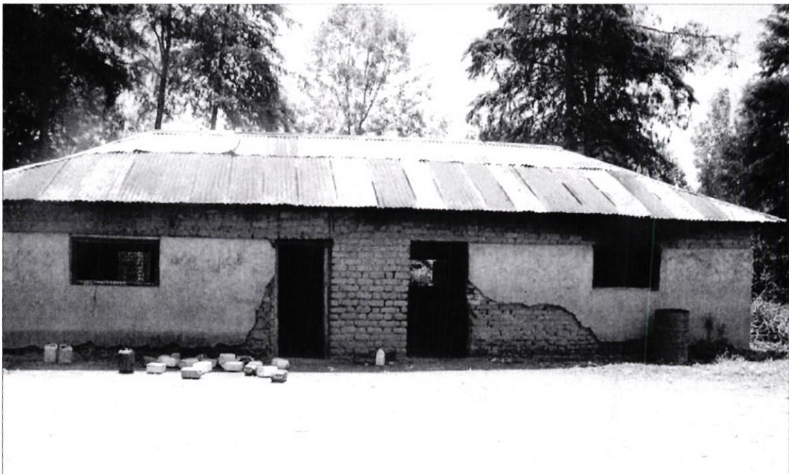
Dilapidated classroom; a common occurrence in many schools.
