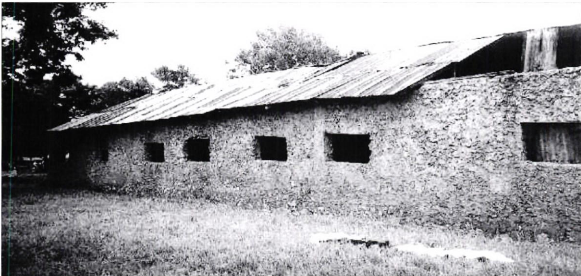
Many schools are in poor condition.
