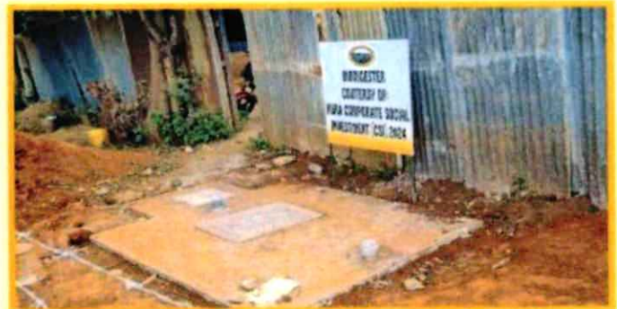
Construction of a Bio-Digester & Soak pit at Tunyai Children Center in Tharaka Nithi County
