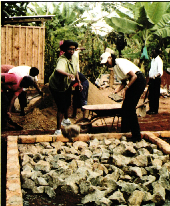
Staff members of ICDCI, in conjunction with Habitat for Humanity Kenya, laying the foundation for a low-cost house in Embu .
