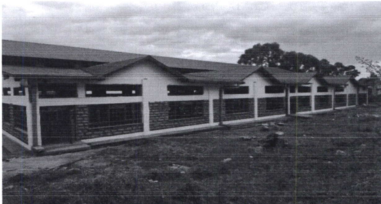
Figure 1: On-going construction of modern 1500 capacity dining hall at Chwele Girls High school
