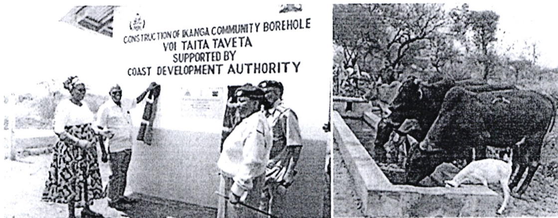
Building communities' resilience against the effects of climate change: Construction of Earth fill pans and drilling of boreholes.
