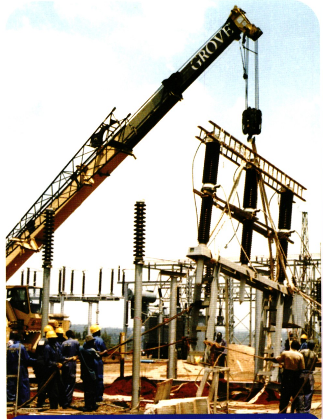
Installation of new equipment at Kiganjo substation has increased its capacity to serve more customers.
