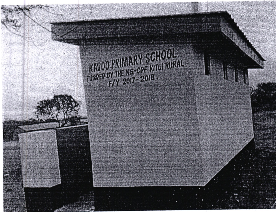
FIG 2.1: Kavoo primary school construction of four door pit latrine FY 2017/18 implemented in 2018/19
