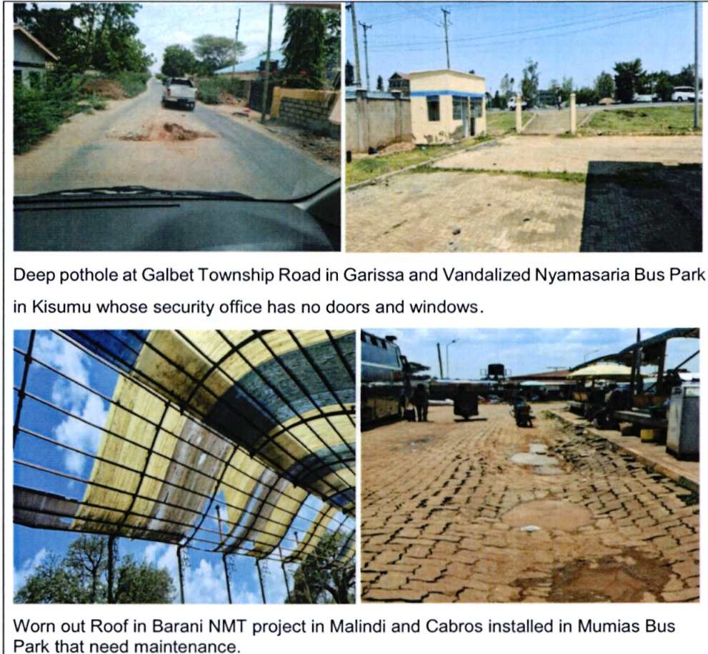
Figure 8: Infrastructure that was in Need of Repairs and Maintenance
