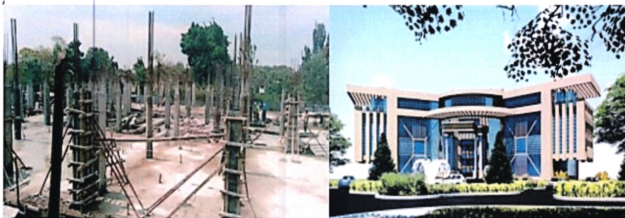
The status of the Modern Administration Block at Main Campus (left) vs the expected block (right).
