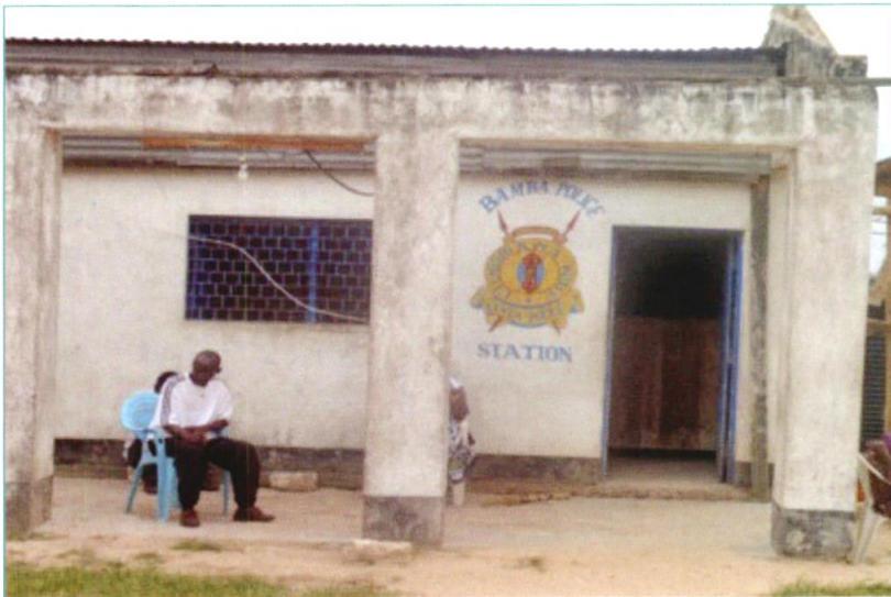
Bamba Police Station lacking a roof
