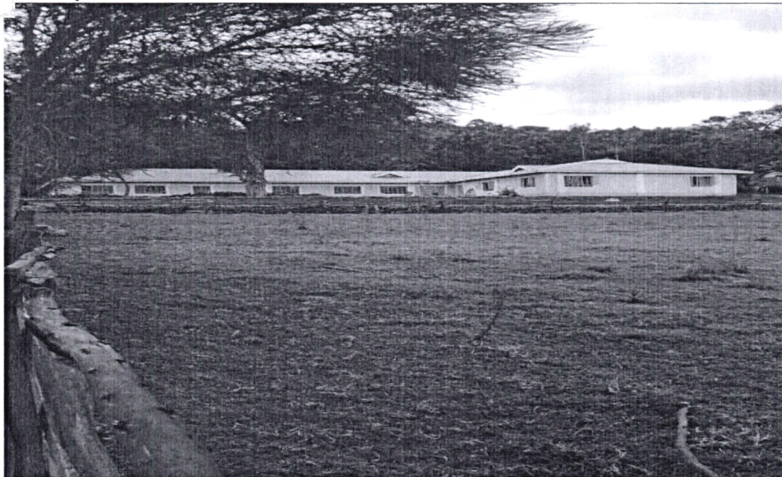
Construction of an administration block at Gonzaga Gonza Secondary School in conjunction with the school PTA
